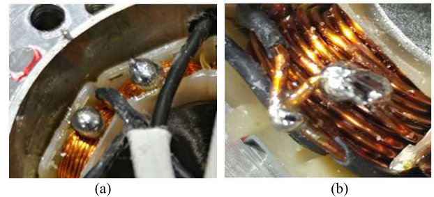
FIGURE 7. Stator winding with ISCF: (a) 100 W and (b) 1 kW.
